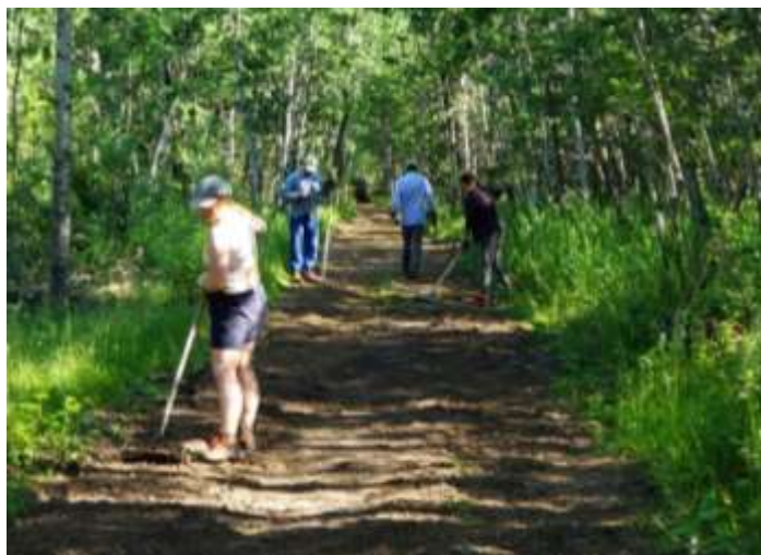
BBO staff and volunteers spread gravel over a deeply rutted section of the access road.
